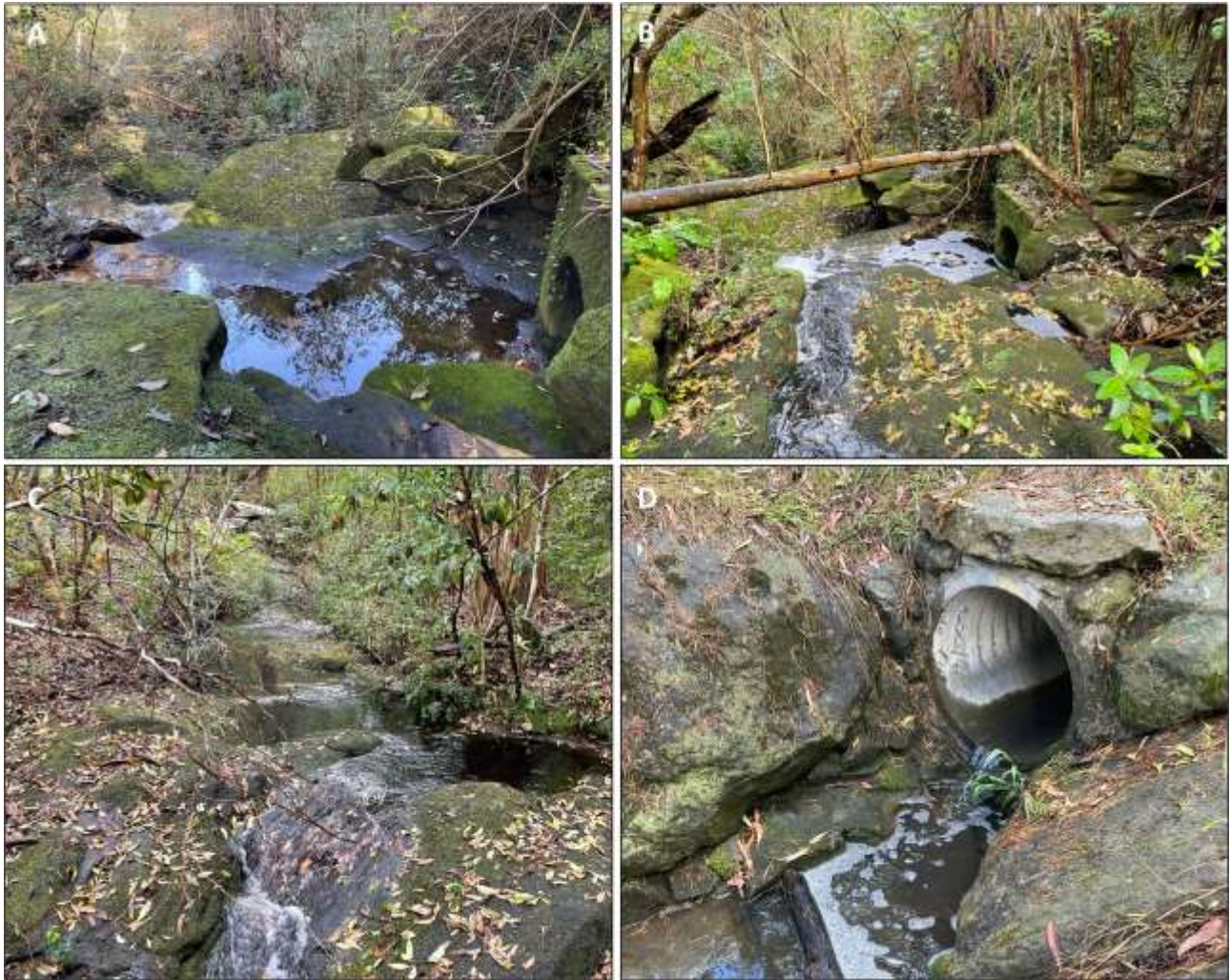
Figure 4-19: Images of Kittys Creek under dry and under a minor storm event
