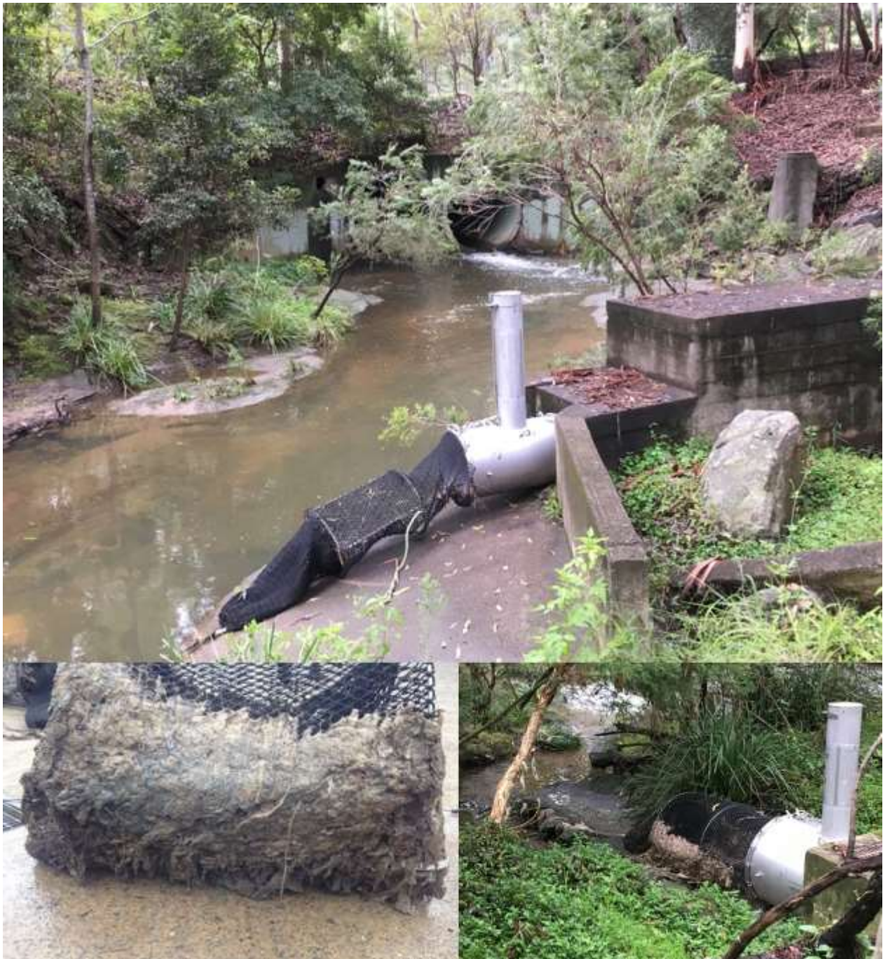
Figure 2-3: Modified Ecosol™ Net Tech trash net attached to sewer overflow structures
