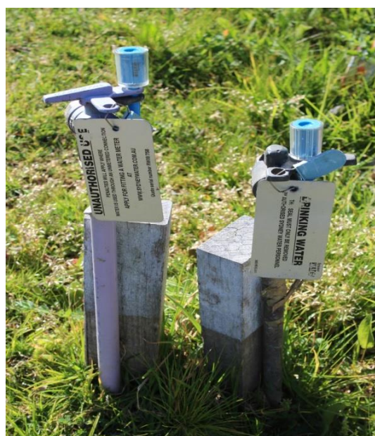
We must install meters for these locked and tagged services.
