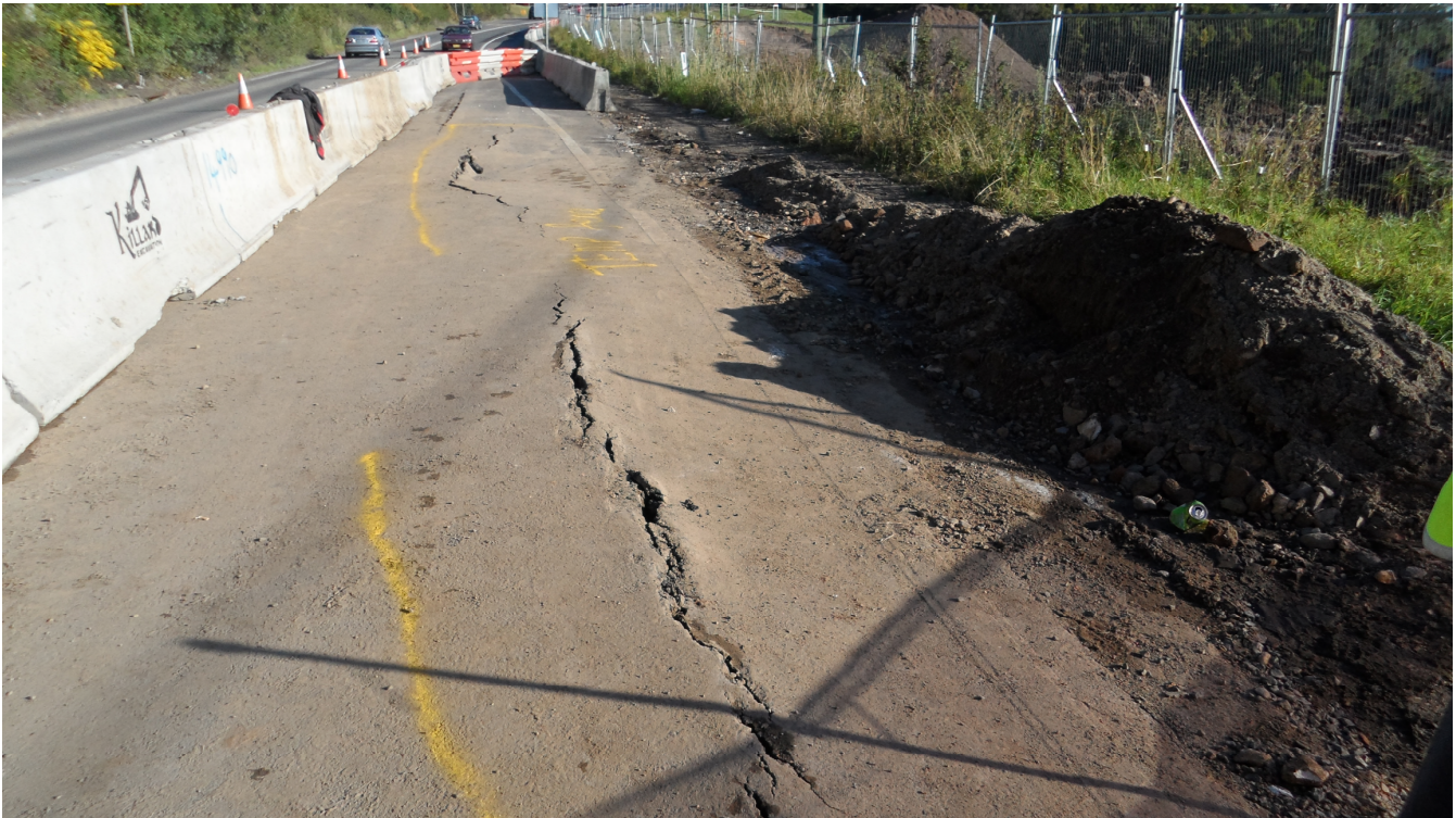
Figure 1: Excessive movement of retaining wall causing road damage and onward failure of water main
