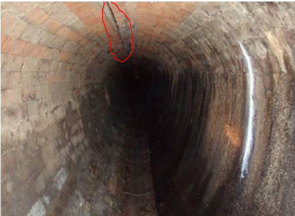
Figure 8: Example of a longitudinal crack in a brick oviform conduit
