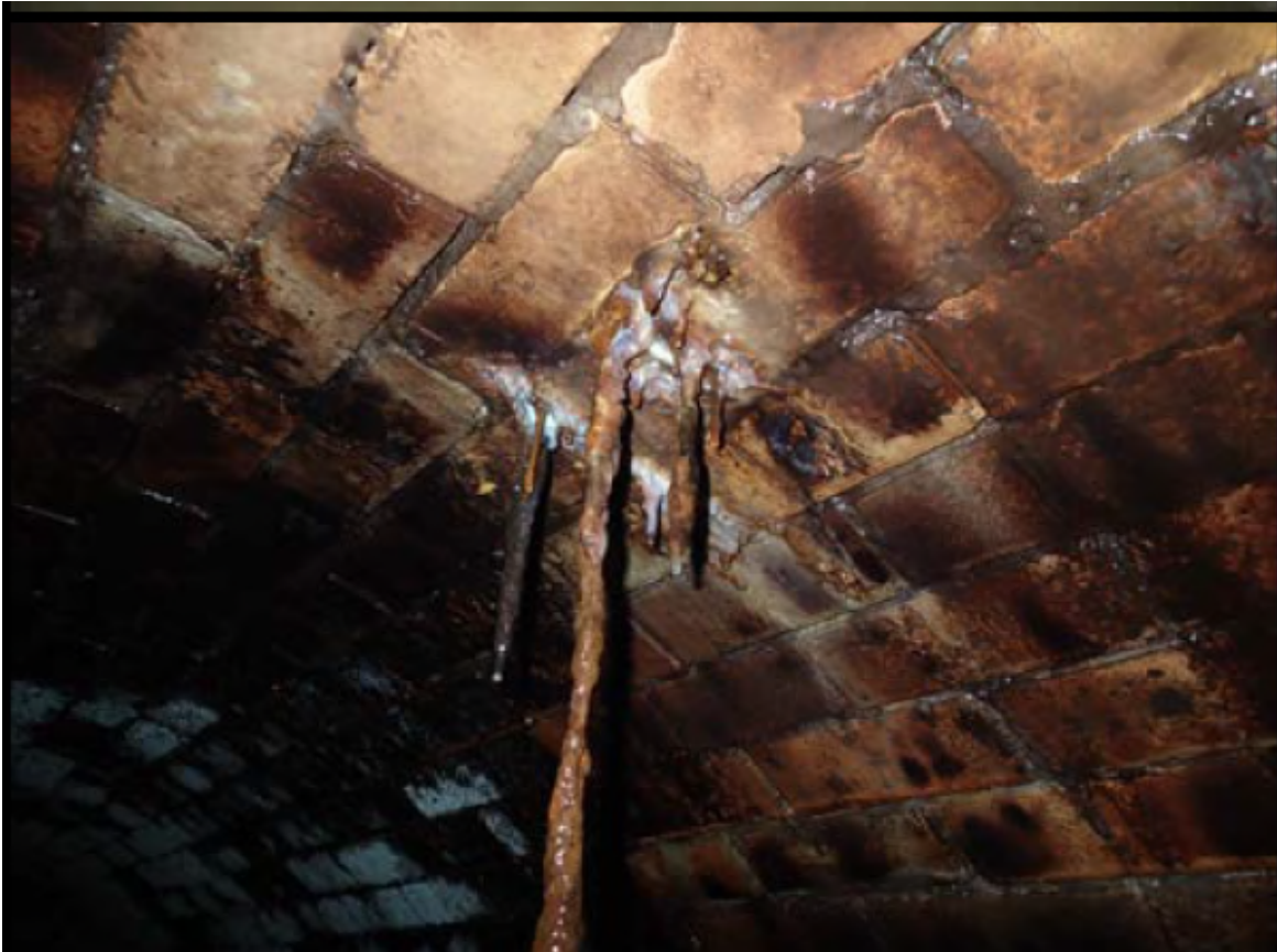
Figure 2: Typical example of infiltration through cracks in a brick oviform
