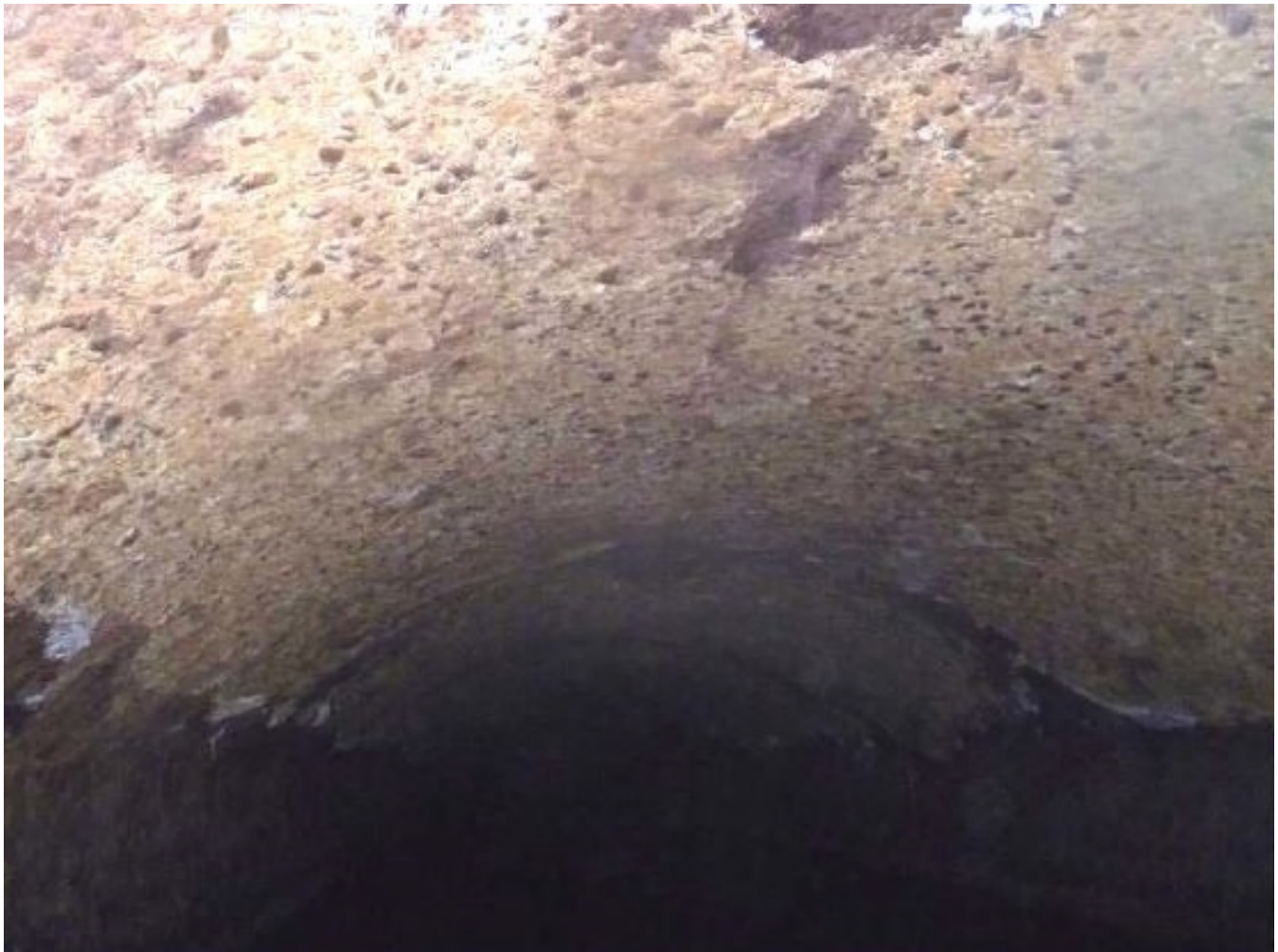
Figure 9: Typical unreinforced concrete lined tunnel showing reduced section
