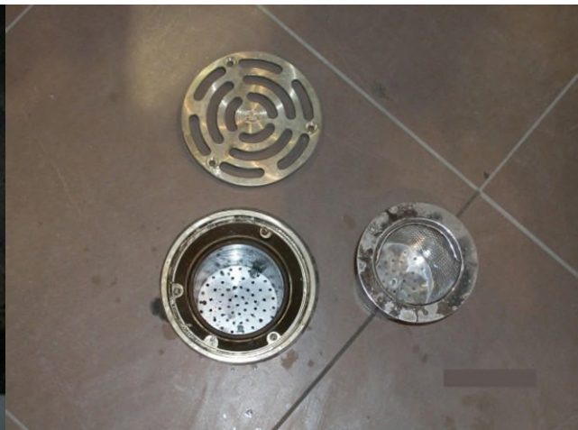
In-floor bucket trap
