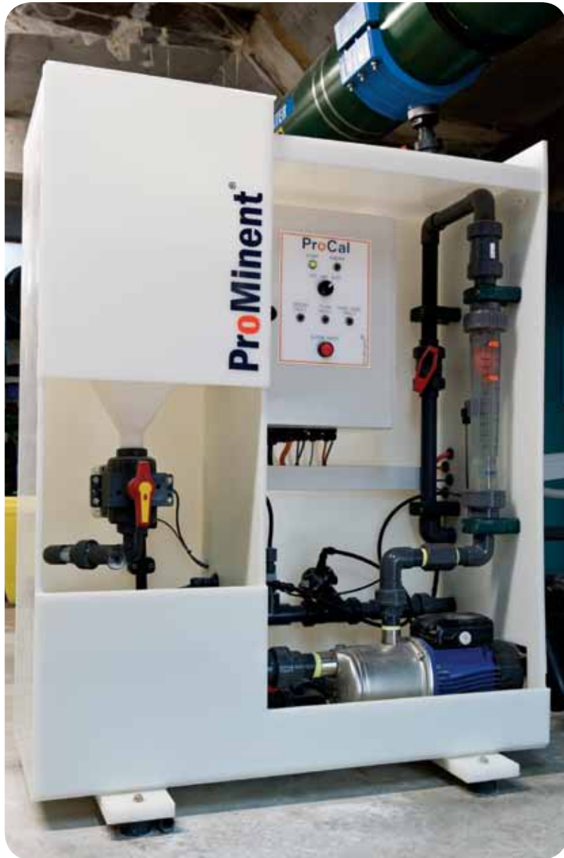
Dry calcium hypochlorite dosing system at Springwood Aquatic Centre. Over the past 10 years, over 300 similar systems have been installed Australia-wide
