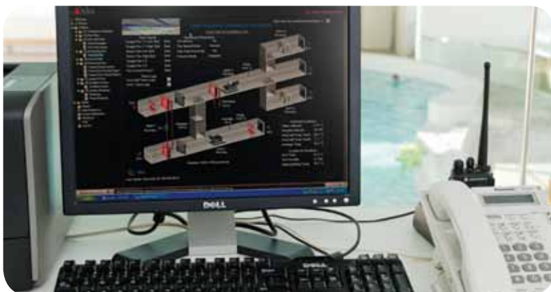
You can use your existing Building Management System to monitor water use by connecting your water meters
