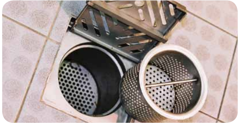
In-floor bucket traps capture food scraps, cutlery and cleaning cloths that may have fallen on the floor. They prevent these items from entering the grease arrestor and encourage thorough cleaning practices
