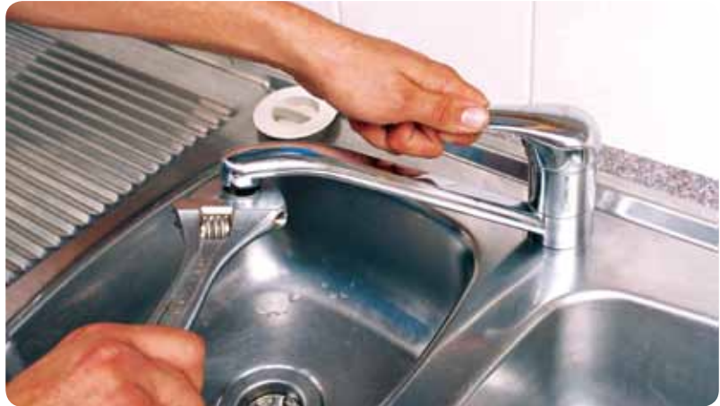
Install flow restrictors on all non-regulated fixtures and repair or replace them as part of an active maintenance program
