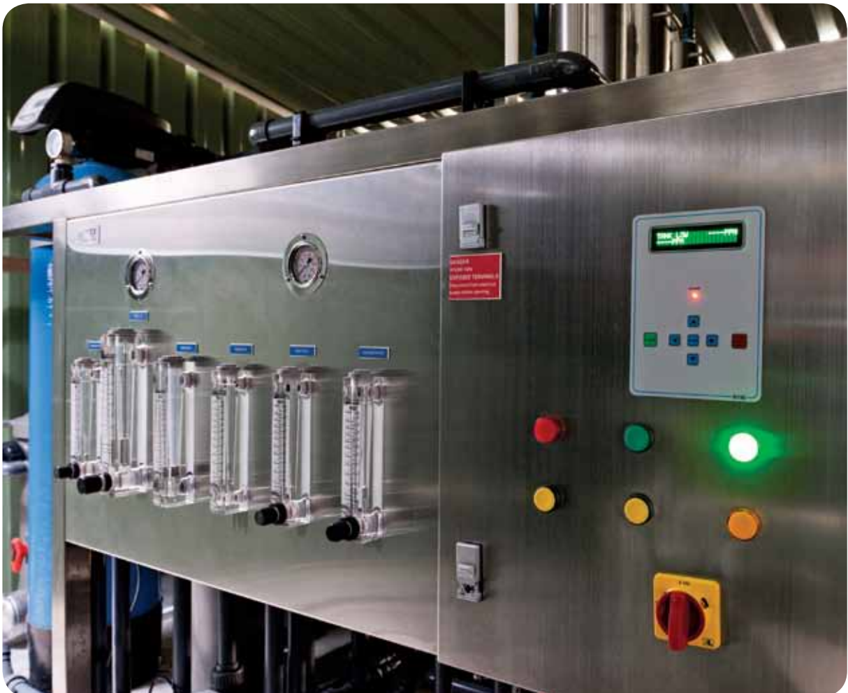
Minimise your water use before considering recycling systems, like this backwash water recycling system at Warringah Aquatic Centre.
