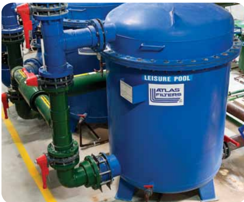
Pressure filters, like this one at Springwood Aquatic Centre are the most common commercial pool filters
