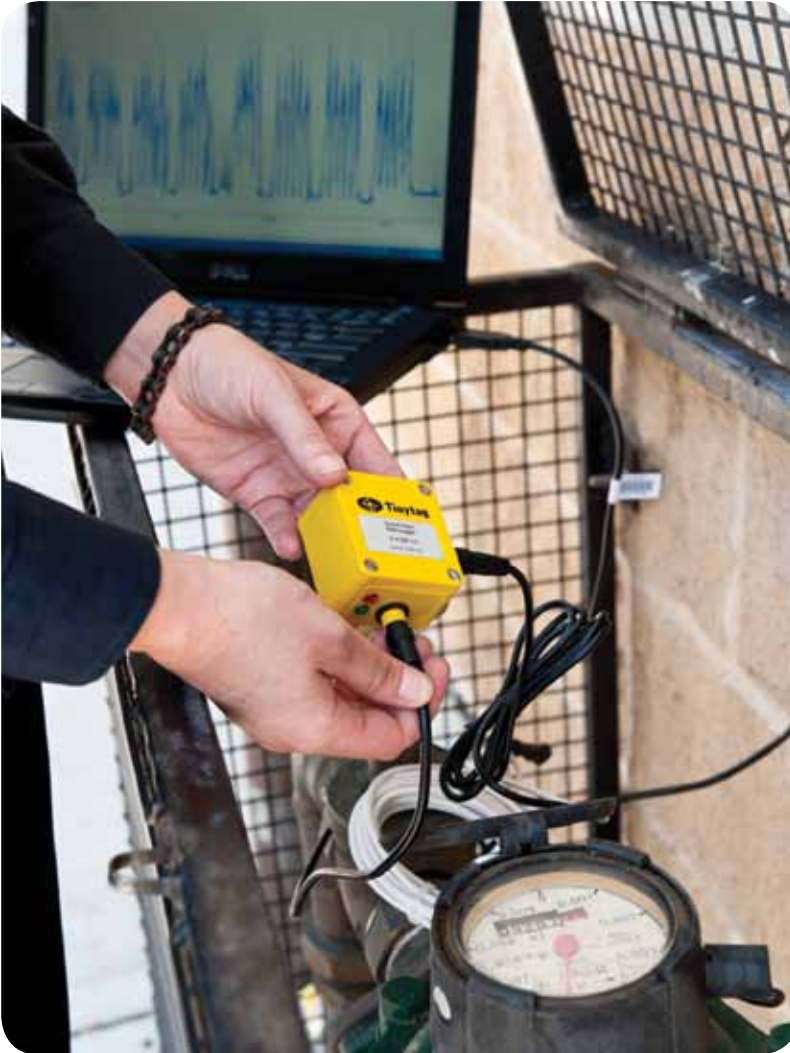
Figure 36 – Data loggers can be easily installed and used
