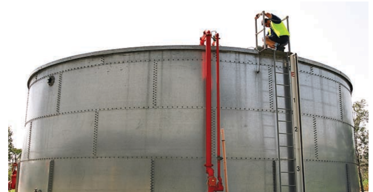
Photograph 11 – Plumbing modifications made by AMP Capital Investors at the Dick Smith Electronic Support Office in the western Sydney suburb of Chullora, allow water used during fire service testing to be captured in holding tanks and reused for later tests. This saves up to 60 kilolitres of water per week.
